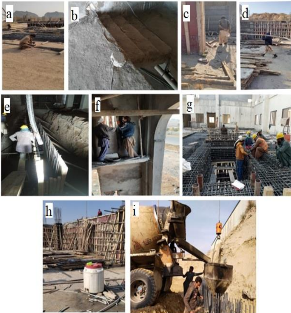
Figure 2: The unsafe work environment that can lead to major accidents or injuries at work sites including Unsafe steel bar cutting (a), Unsafe electricity connection (b), Unsafe extension cords (c), Unsafe manual lifting (d), Poor lighting (e), No PPEs (f), Non-Compliance of Covid SOPs (g), Unhygienic water coolers (h), and Unsafe Excavation work (i) The worksite operated during the night lacked sufficient lighting, making it difficult for workers to see clearly and navigate safely, as seen in Figure. 2(e). Moreover, the majority of workers on the site were not provided with Personal Protective Equipment (PPE), as shown in Figure. 2(f), putting them at risk of injury or illness. Despite the ongoing COVID-19 pandemic, it was observed that the recommended standard operating procedures (SOPs) to prevent the spread of the virus were not being followed on the site, as illustrated in Figure. 2(g). Most construction sites lacked a safe drinking water facility, and the available water coolers, as shown in Figure. 2(h), were often unhygienic. Moreover, the coolers were not easily accessible to the laborers working at heights, posing a risk to their health and safety.
